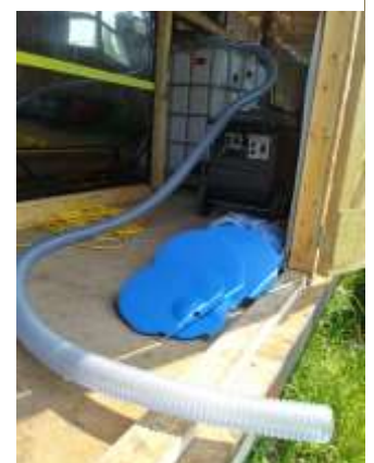
Figure 20.1: Hose leading outside
